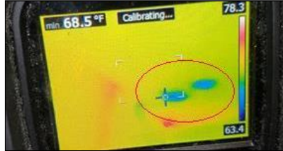
3.1 Item 2(Picture) Thermal imaging – tested elevated – Observed in- unit 3 bathroom
