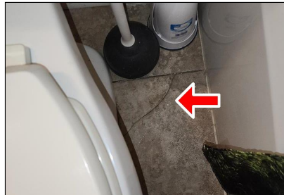
3.0 Item 11(Picture) Example/ Sample- 8- Bathroom
