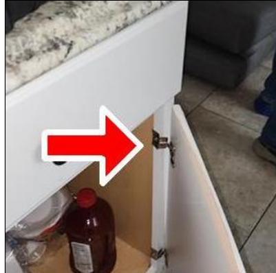
3.4 Item 2(Picture) Example/ Sample- 8- Kitchen- loose hardware
