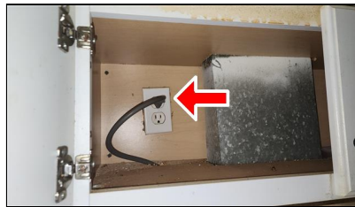
6.4 Item 5(Picture) Example/ Sample- 4- Kitchen- Loose junction box
