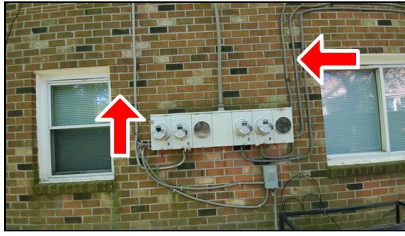
2.0 Item 8(Picture) Example example rear of building cracking
