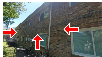
2.0 Item 7(Picture) Example/ Sample- Rear of building – cracking
