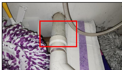
5.4 Item 4(Picture) Example/ Sample- 7-Kitchen Sink- appears to be PVC to ABS connection made with glue/solvent
