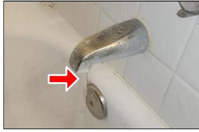
5.4 Item 8(Picture) Example/ Sample- 6 Bathroom Shower- tub spout leaks when in shower mode (this waste supply water, and could affect shower water supply)
