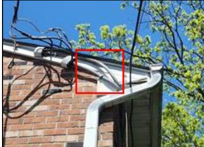
6.2 Item 1(Picture) Example/ Sample- electrical service conductors are frayed at wire sheathing
