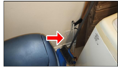
6.4 Item 3(Picture) Example/ Sample- 3- Living Room- loose outlet
