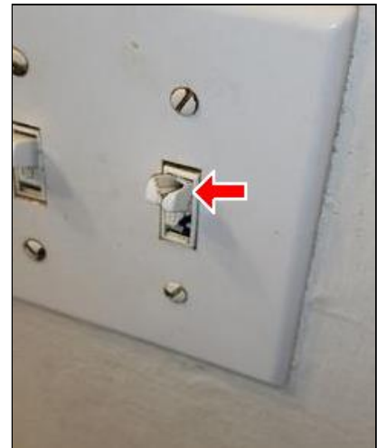
6.4 Item 6(Picture) Example/ Sample- 2- Bathroom- Damaged switch
