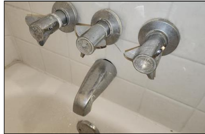
5.4 Item 9(Picture) Example/ Sample- 2- Bathroom Shower- plumbing tree component is loose, gap at tub spout, crack/ damage tile
