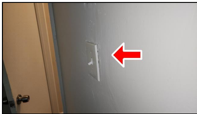
6.4 Item 4(Picture) Example/ Sample- 3- Rear Left Bedroom- Loose switch
