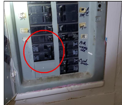
6.3 Item 3(Picture) Main cut off week relocated in the panel which is considered acceptable however cut off breaker not attached with screw – Example/Sample-unit 3
