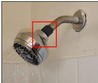
5.4 Item 1(Picture) Example/ Sample- 7- Bathroom Shower shower heads leaks
