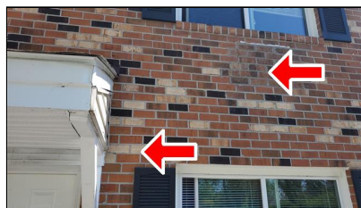
2.0 Item 6(Picture) Example sample front of building – cracking
