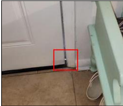
3.2 Item 1(Picture) Example/ Sample- Front Door 7- Exterior door(s) – weather-stripping- missing
