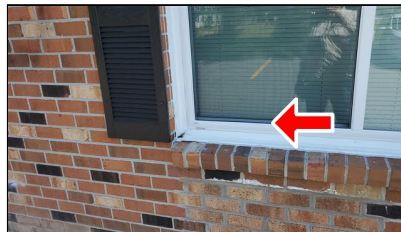
2.0 Item 2(Picture) Example sample front of building –window sill slope improper – at least keep this area caulked to prevent water entry
