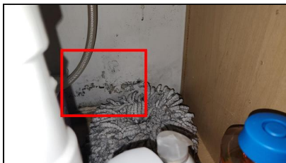
3.1 Item 4(Picture) Example/ Sample- 7- Kitchen Sink
