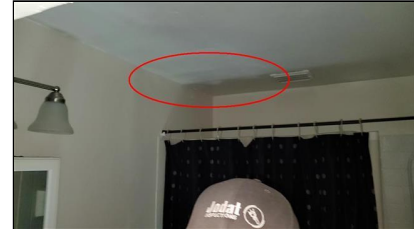
3.1 Item 3(Picture) Thermal imaging – tested elevated – Observed in- unit 3 bathroom
