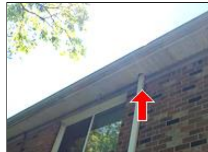
2.0 Item 3(Picture) Example/ Sample- rear of building – openings, loose soffit
