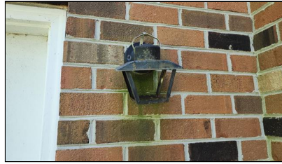
6.5 Item 2(Picture) Example/ Sample- Left side of Building- Damaged, bulb missing
