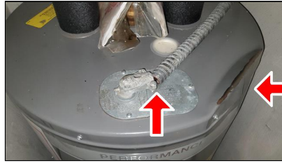
5.5 Item 2(Picture) Example/ Sample- unit 6
