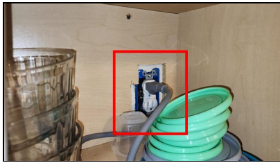
6.4 Item 1(Picture) Example/ Sample- 7- Kitchen- cover plate missing
