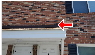
1.0 Item 2(Picture) Example/ Sample- front of building – slightly lifted risen flashing
