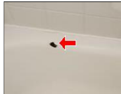
5.4 Item 3(Picture) Example/ Sample- 7- Bathroom Shower-tub finish damage
