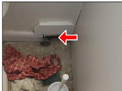
5.2 Item 2(Picture) additional water cutoffs located in 2-Bathroom
