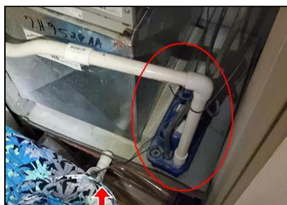
7.2 Item 2(Picture) Example/ Sample- float switch, and condensation pump
