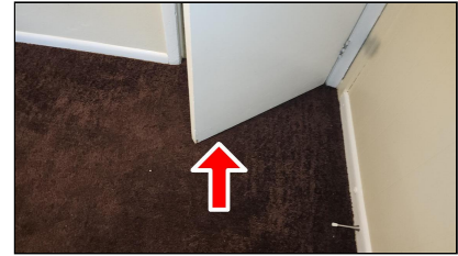
3.2 Item 3(Picture) Example/ Sample- 6- Rear Right Bedroom- Rubs the floor
