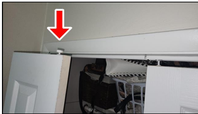
3.2 Item 4(Picture) Example/ Sample- 1- Rear Right Bedroom Closet- sliding door does not stay in track
