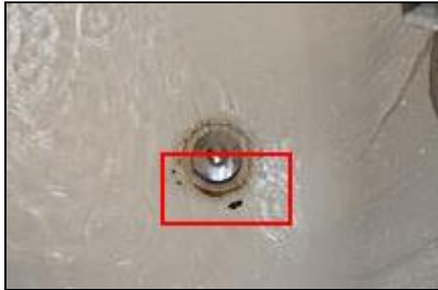
5.4 Item 7(Picture) Example/ Sample- 6 Bathroom Shower- tub finish damage that appears to be a cosmetic concern
