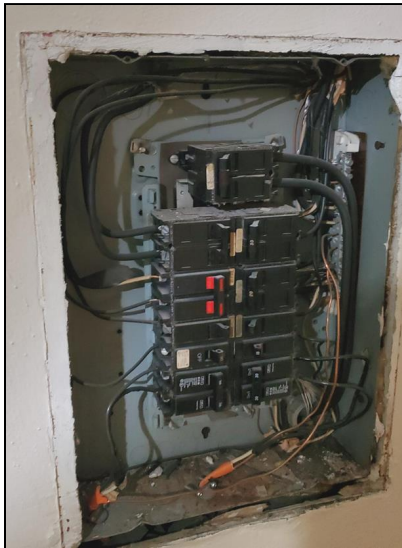
6.3 Item 1(Picture) Example/ Sample- unit 7 – panel uncovered by inspector during inspection process
