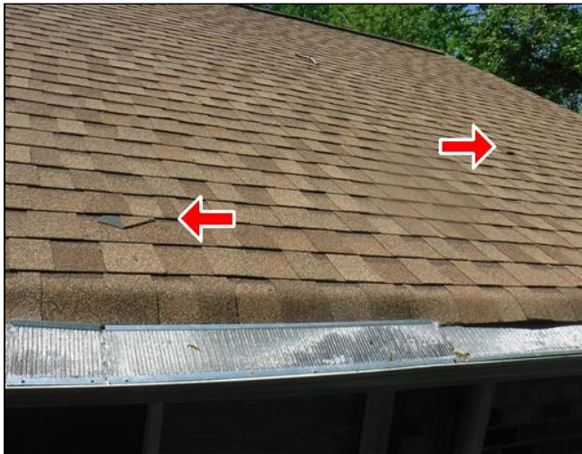
1.0 Item 3(Picture) Example/Sample- rear of building – lifted risen shingle, damaged shingle
