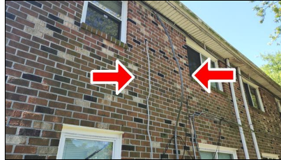
6.2 Item 2(Picture) Example/ Sample- Service entrance ca ble straps missing and/or not supported properly
