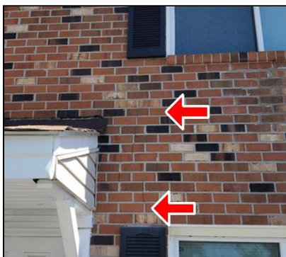
2.0 Item 5(Picture) Example/ Sample- front of building front of building – near the right side cracking
