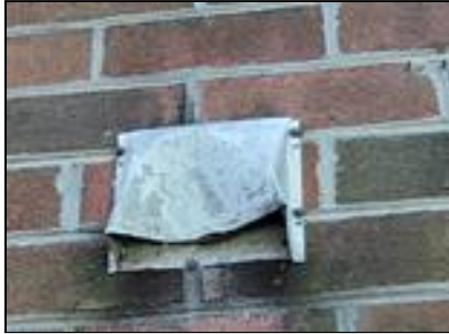
8.3 Item 1(Picture) Example/ Sample- one of multiple that are damaged/dented
